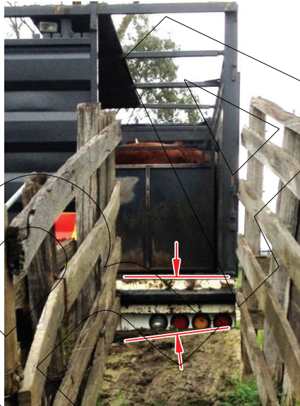
Figure B.3(F) — Poor alignment of ramp to livestock crate floor
