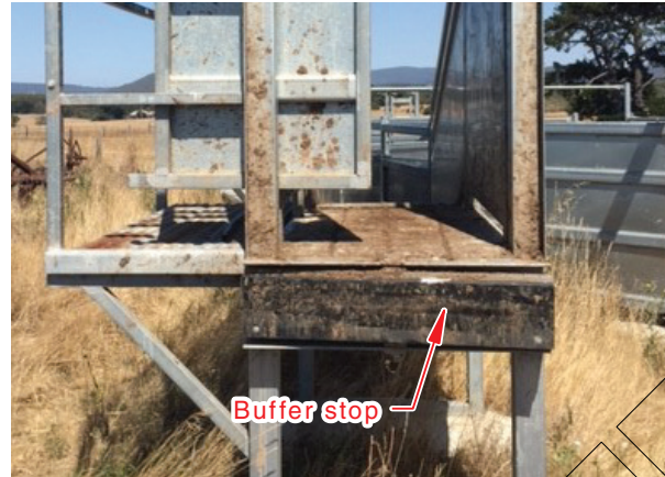
Figure B.3(G) — Buffer stop on front of ramp in good condition
